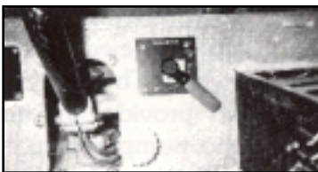
Heater ON/OFF valve
