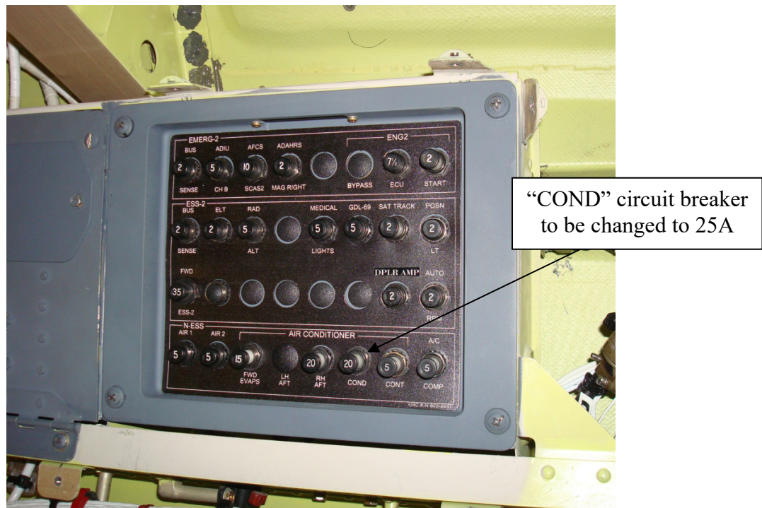
Figure 4. Circuit Breaker panel
