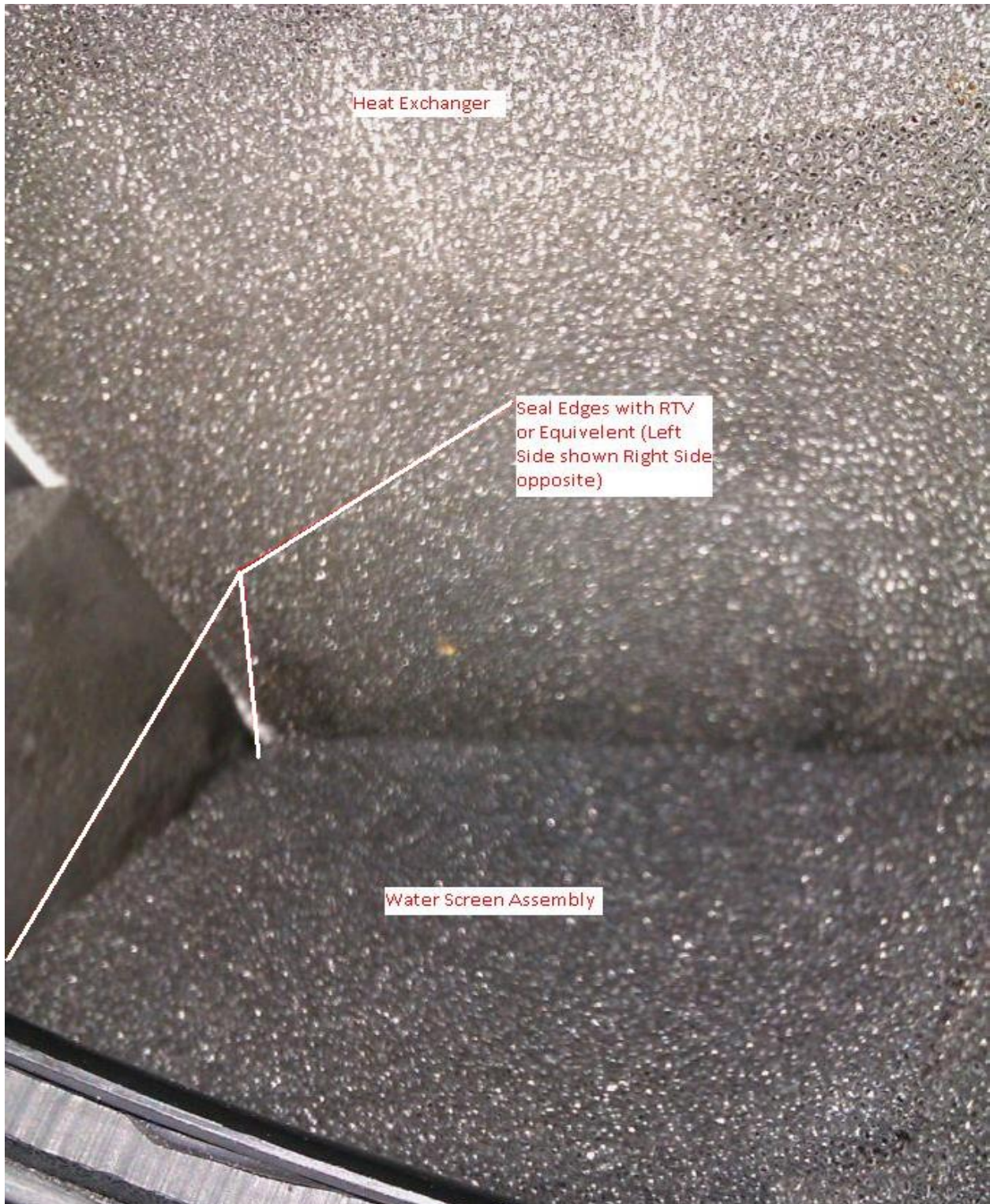
Figure 14: 429EC-6242-1 Water Screen Assembly Installed
